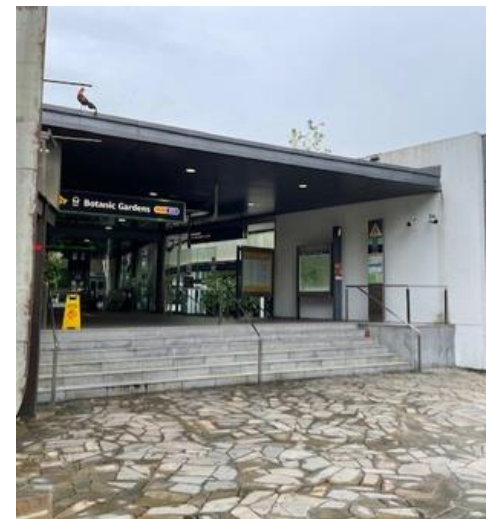
Eaves of entrance is too short and attracts rainwater
