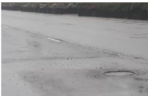
Figure 1: Illustration of pothole on roads.
