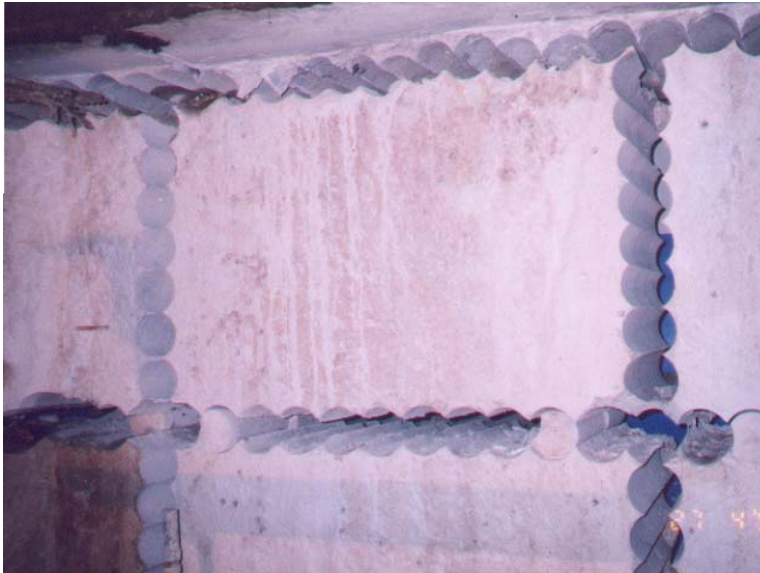
Figure 2-12 Stitch coring method for cutting wall panels helps to minimise vibration and noise levels
