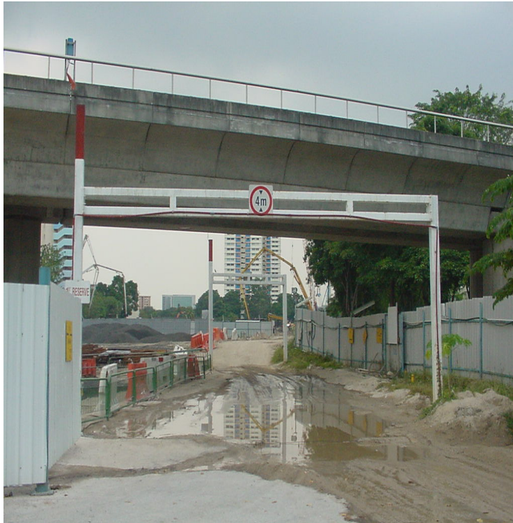
Figure 2-10 Temporary height restriction gantries are provided on both sides of the viaduct beam
