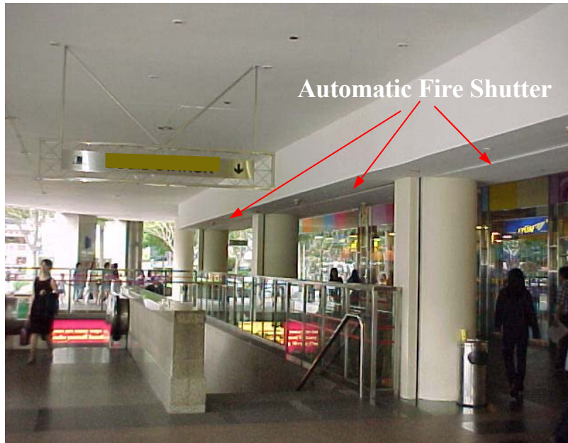
Figure 4-35 An automatic fire shutter at the interface between a commercial development and station entrance
