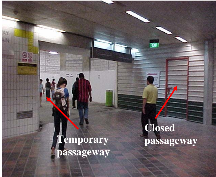
Figure 2-9 A safe and protected temporary passageway is provided during the construction of a commercial development
