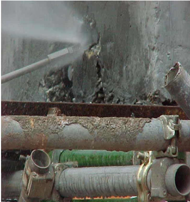
Figure 2-15 Use of a hydro-jet for demolition helps to minimise dust, fire hazard, vibration and noise levels
