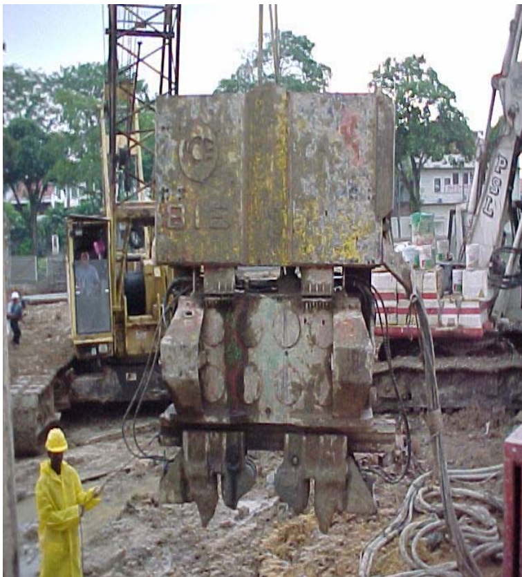
Figure 3-8 View of a vibro-hammer
