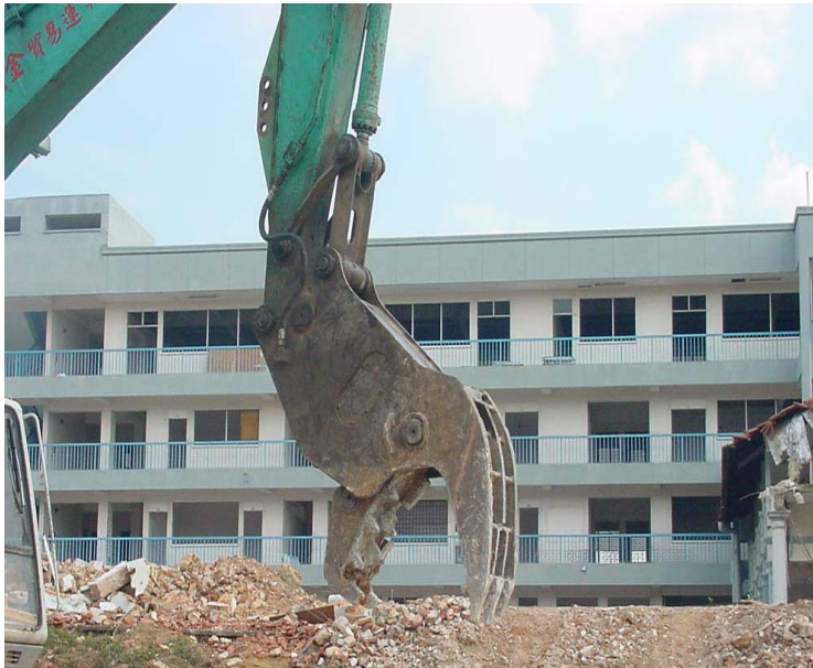
Figure 2-11 Use of a crusher for demolition helps to minimise the impact of vibration
