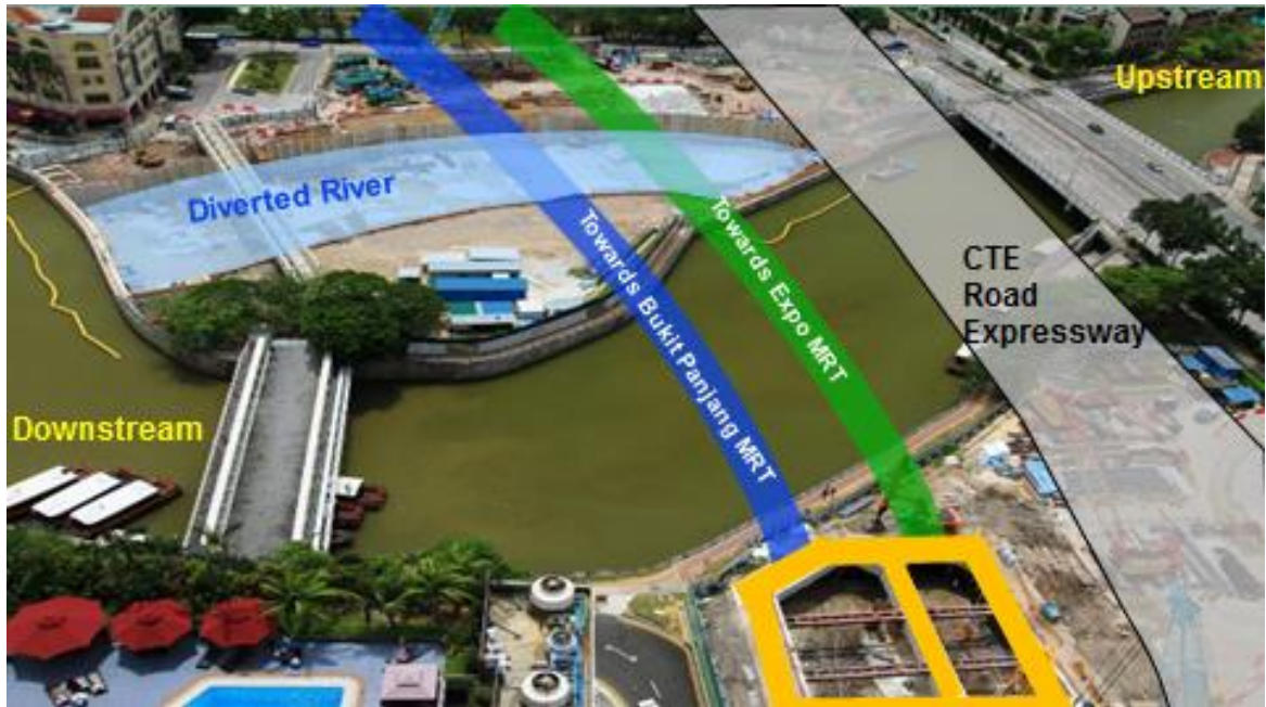
Picture A: Construction of Fort Canning Station and Tunnels in Singapore – Singapore River diverted
