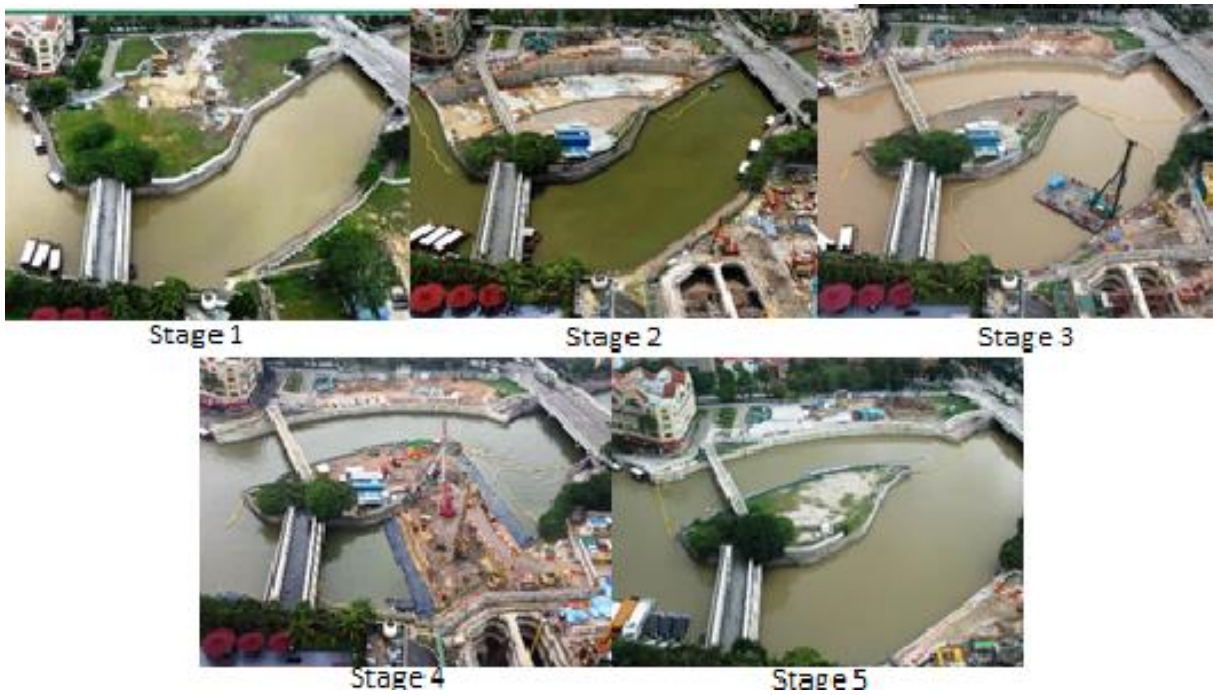
Picture B: Construction of Fort Canning Station and Tunnels in Singapore – Singapore River diverted and original waterway later reinstated
