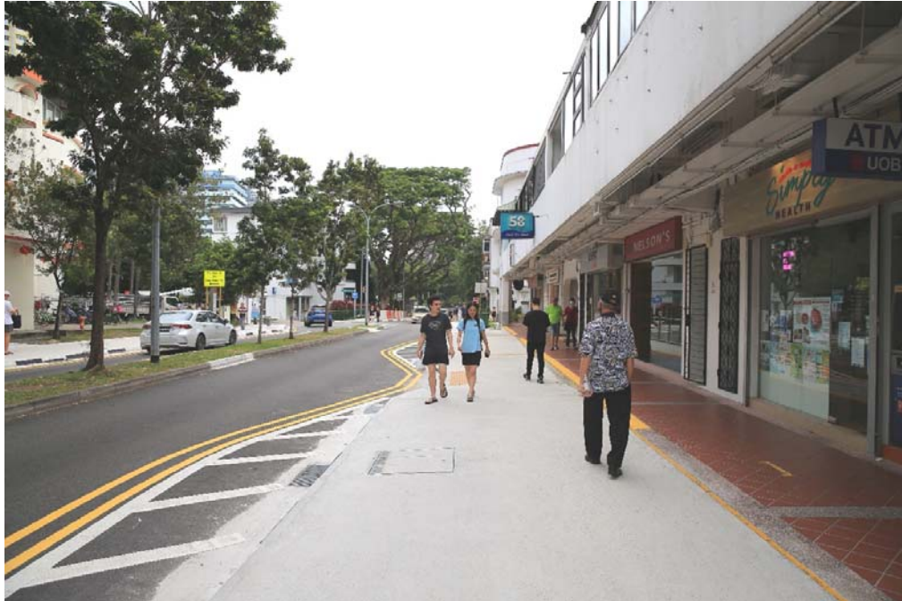
After: Widened footpath and new barrier-free access ramp along Seng Poh Road
