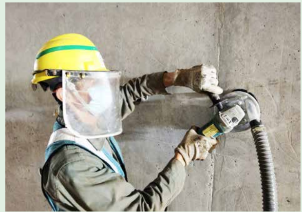
Dust vacuum system implemented at project sites to minimise dust accumulation
