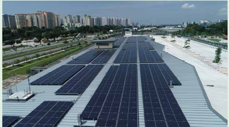
Solar PV systems installed at Gali Batu Integrated Depot
