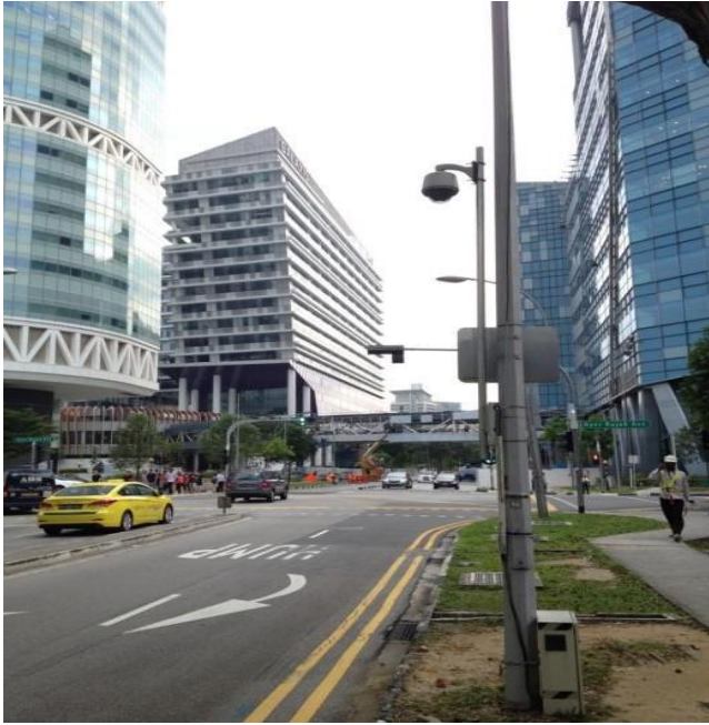
CCTV camera installed at the junction of Fusionopolis
