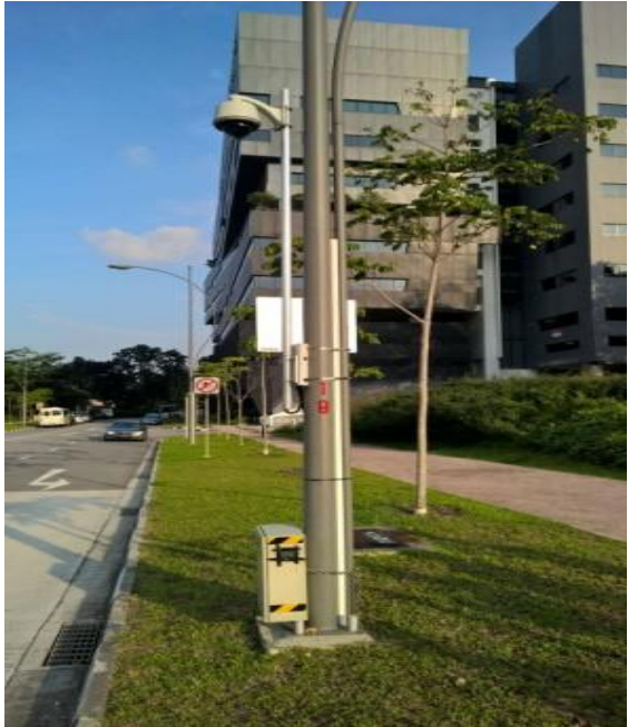
CCTV camera installed at Media Circle
