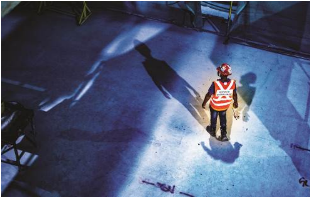
The Road to the Future Is Under Construction by Lim Mark Anthony Pamintuan
